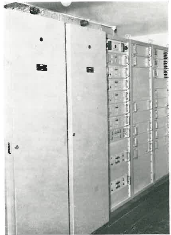
Figure 5 On the left are two racks each containing twenty 5kW dimmers. The three cabinets on the right contain the magnetic memory and electronic control equipment.
